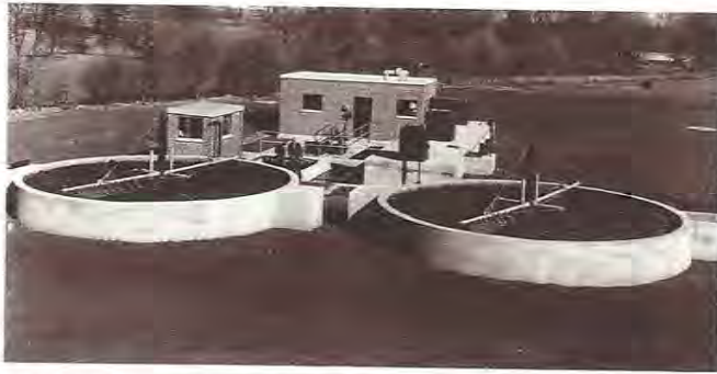
Apartment complexes, shopping centers, camps, and similar properties will sometimes have a small sewage treatment plant on their grounds. This type of plant operates on the same principles as an activated sludge plant, only on a smaller scale.
